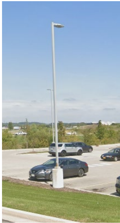
Lighting at 111 E Wolf Run
