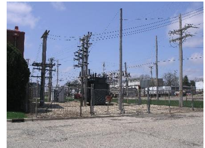
Electric substation in the City of Elkhorn
