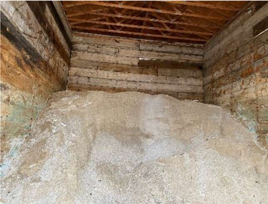
Sand Shed rotting (demolish)
