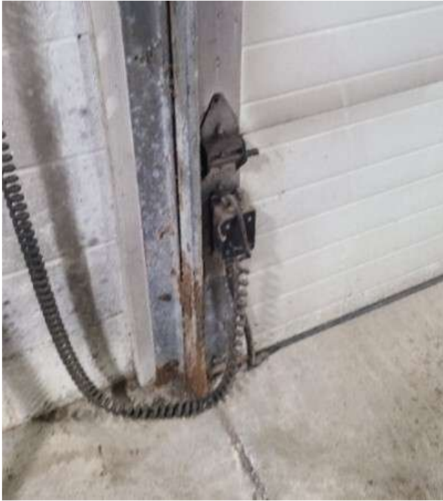
Deterioration on overhead door from Salt Brine
