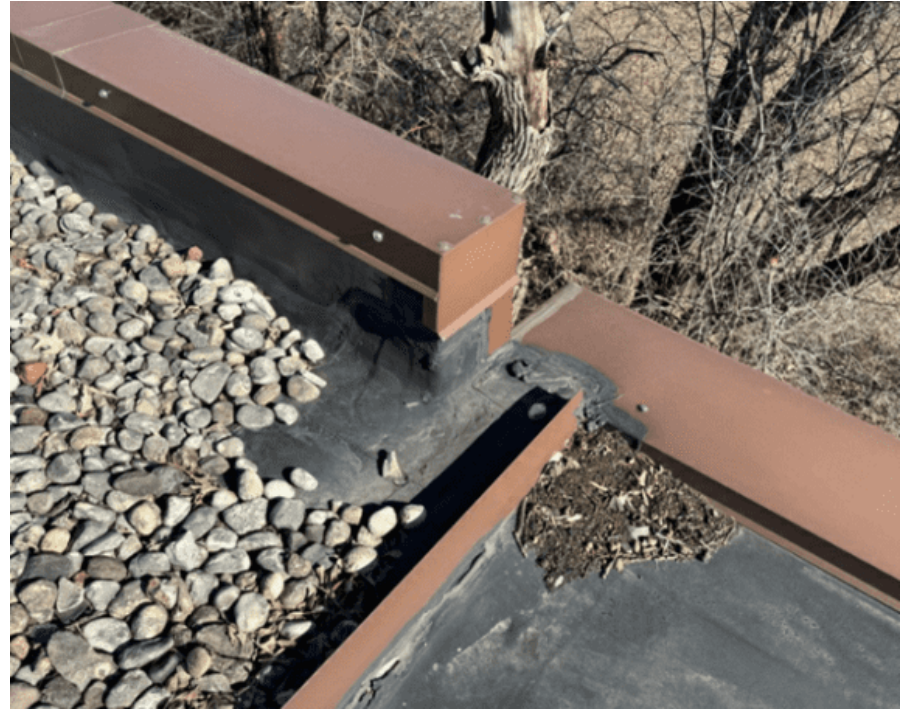
Improper detailing & waterproofing
