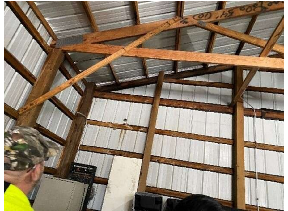
Impound storage structure is rotting & metal is damaged (demolish)
