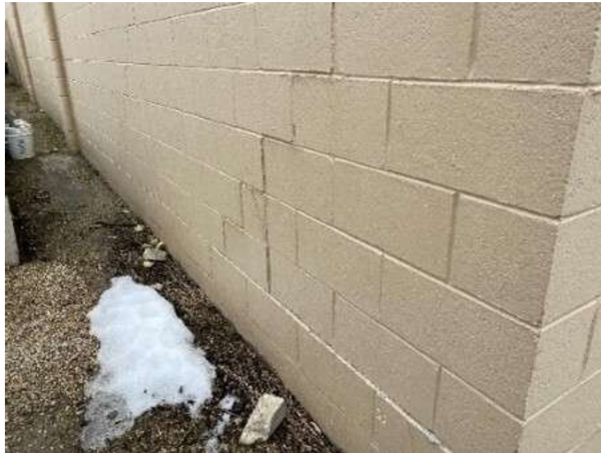
Settlement (Parking Garage)
