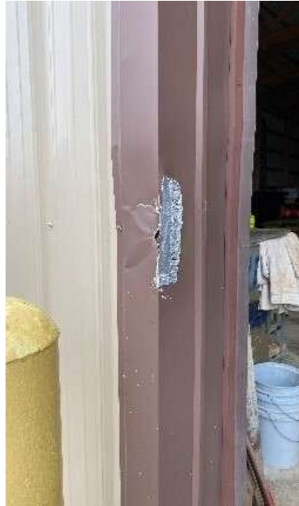
Damage from Trucks
