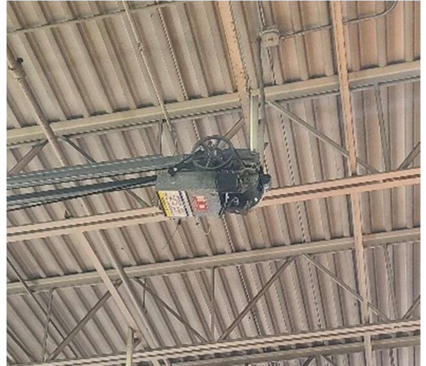
Damage on garage opener from low ceiling
