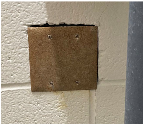
Photo 4, Electrical junction box exposed to fluoride
