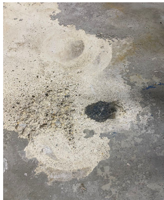
Photo 6, Concrete exposed to fluoride
