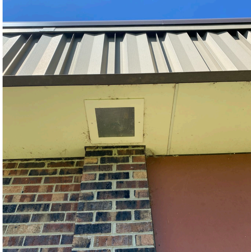
Outdated Site & Building Lighting
