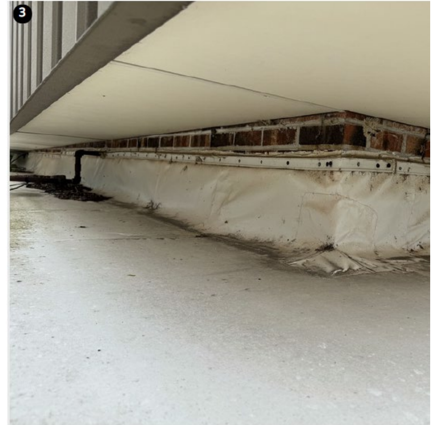
Improperly Secured and Sealed Flashing
