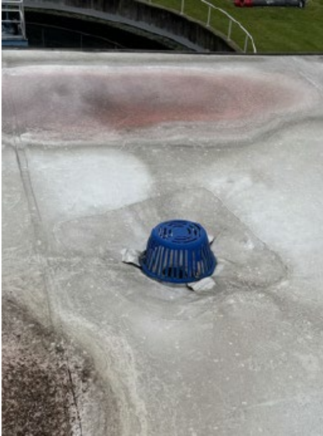
Improper Drain Detail Drain is loose
