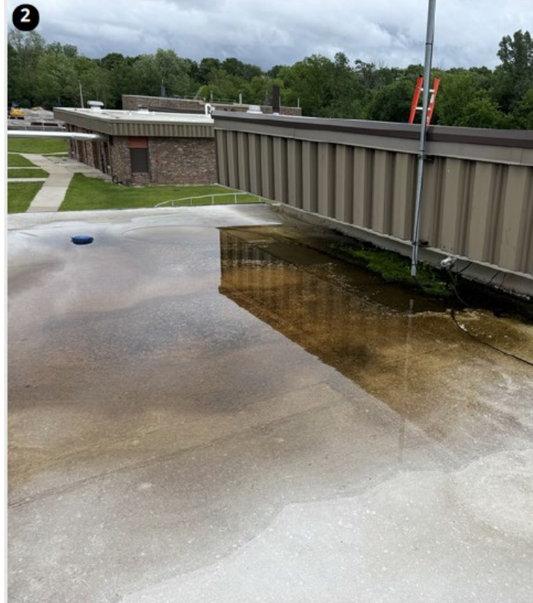
Roof Ponding (Clogged Drain)
