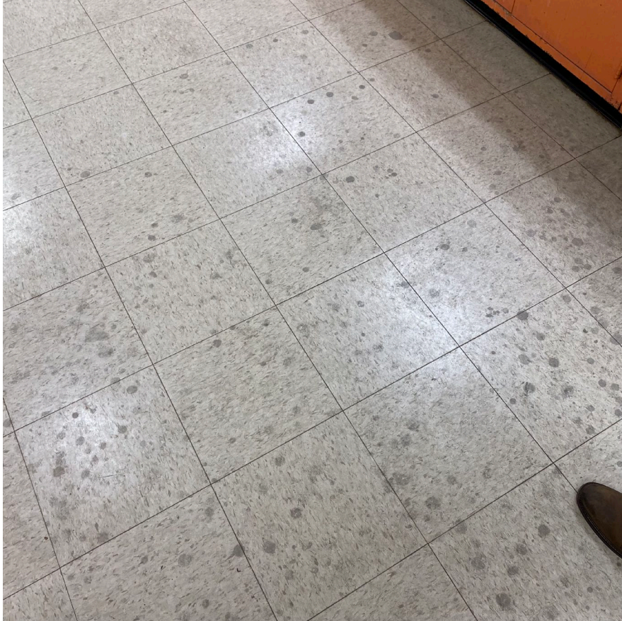
Acid Damage from Lab (Ceilings and Floor)
