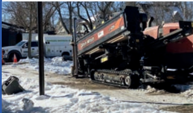
Fiber optic cables being laid underground on the south side of the building
