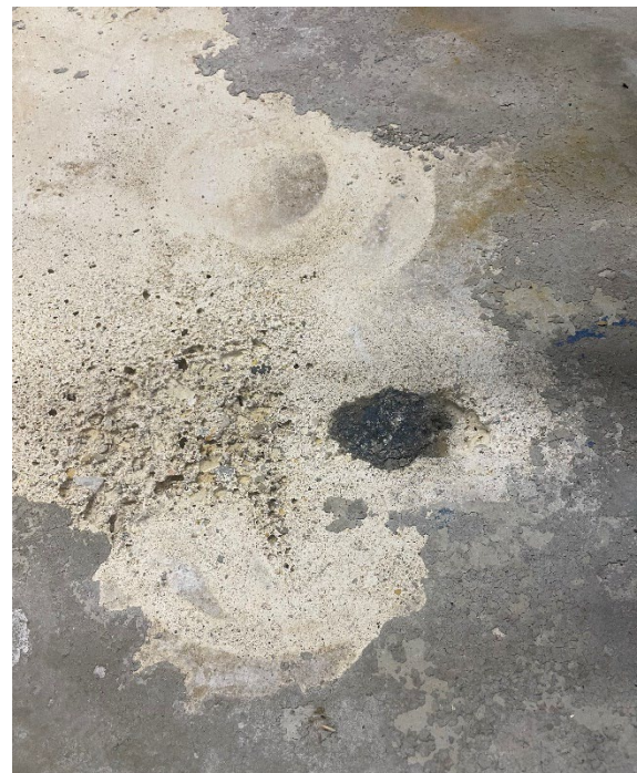
Photo 6, Concrete exposed to fluoride
