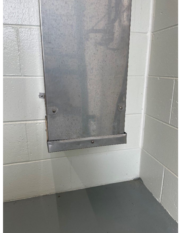
Photo 5, Vent not exposed to fluoride
