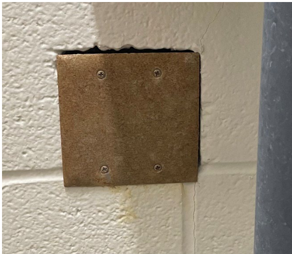
Photo 4, Electrical junction box exposed to fluoride
