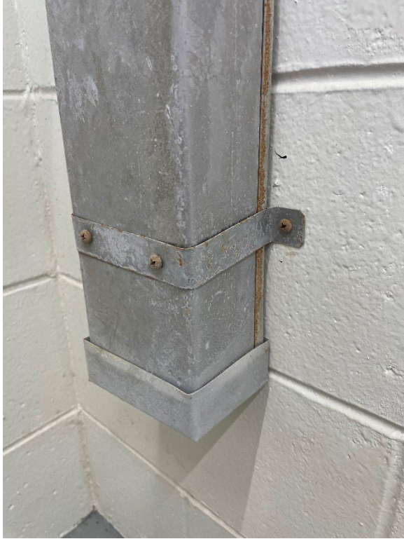
Photo 3, Vent exposed to fluoride
